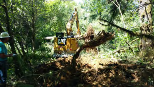
A backhoe lifts a fallen tree, preparing it for placement into Ritner Creek
