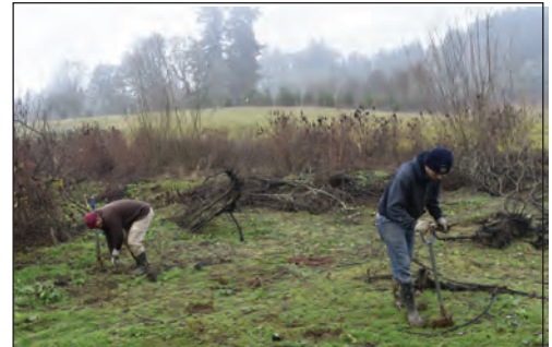
D. Franco Contracting, Inc. crewmembers plant live cuttings within a newly constructed swale at the LSNA Floodplain Reconnection Project site.
