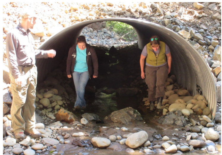
The new culverts are much bigger and embedded into the stream bed, allowing fish—including coho, lamprey, steelhead and cutthroat trout—to migrate further up the creek.
