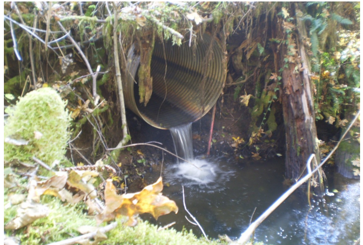
Undersized culverts on Price Creek presented a barrier to native salmon and trout trying to access prime upstream habitat.
