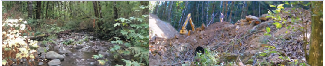
(L) Located in the upper part of the watershed, South Fork Pedee Creek is a tributary of mainstem Pedee Creek, which in turn, flows into the Luckiamute River. (R) Construction crews begin work to replace an undersized and perched culvert with a properly sized one, which will result in both immediate and long term benefits to native fish and other aquatic life.
